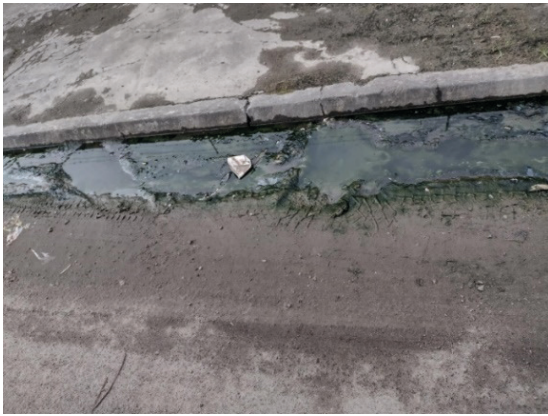
Figure 12 - Streets with open sewers
